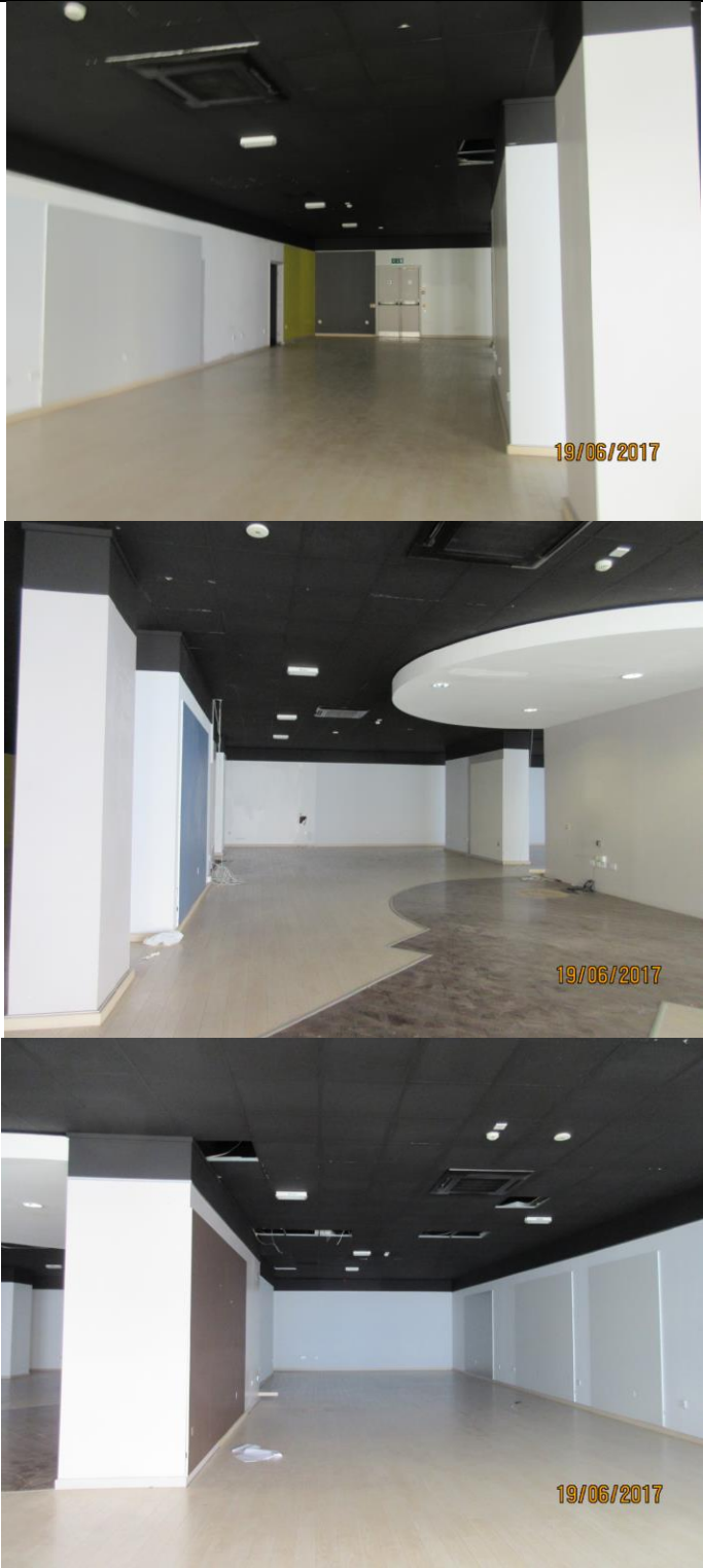
Photos of the inside of the triple unit, showing each of three areas with dividing walls
